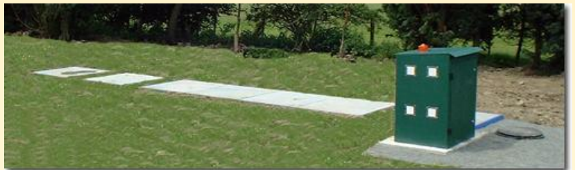
200 Population equivalent installed. Showing finished landscaping, control kiosk with air louvers and loss-of-air alarm beacon.
